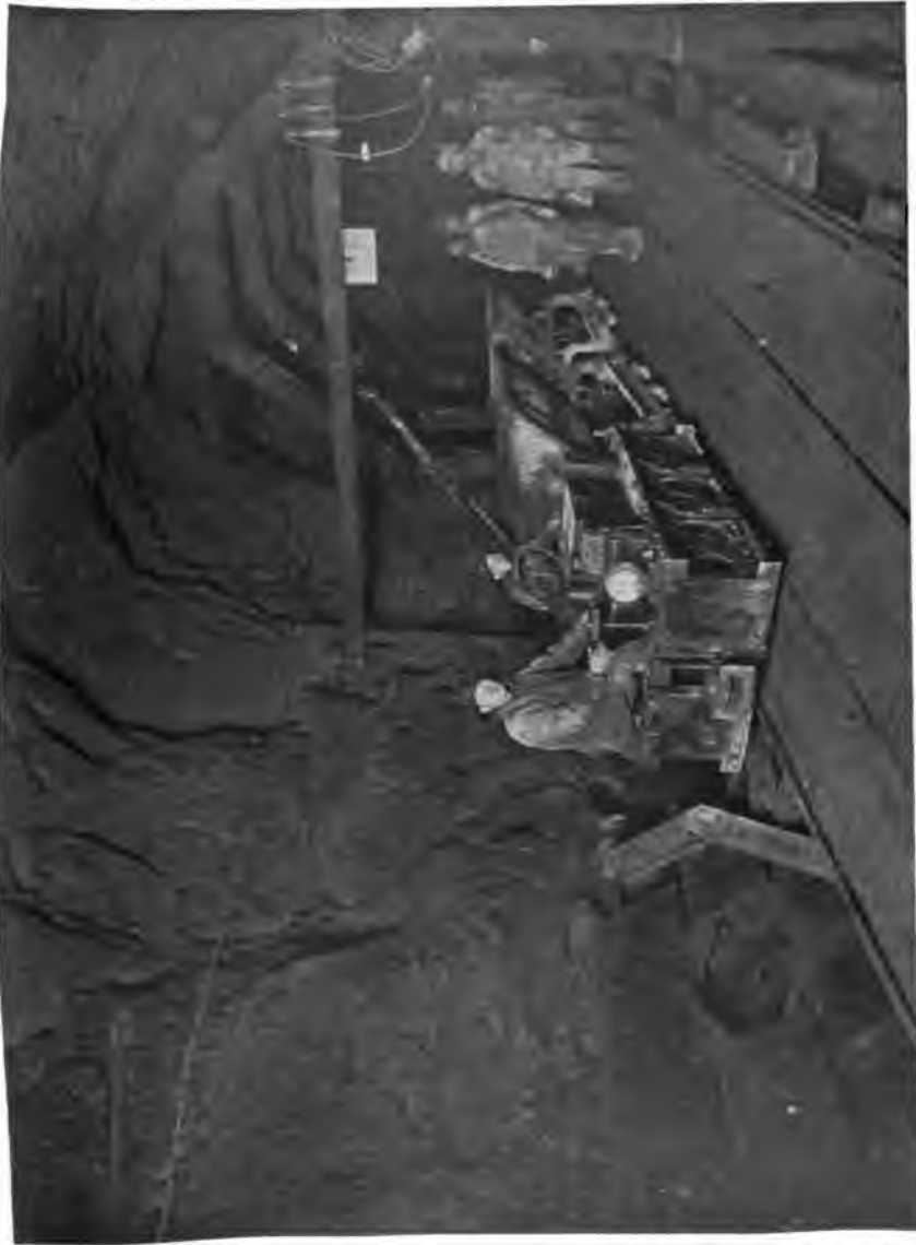
PLATE 121.—Contract 47. Electric Trolley Locomotive Used for Hauling Concrete for Lining Walkkill Tunnel. These locomotives enabled much better progress to be made than where mules were used.
